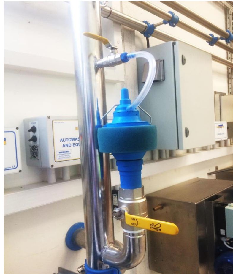
Regulator(s) plugged (fully isolate)
