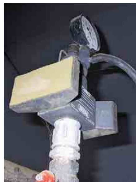
Regular cleaning of the filters on the vacuum regulator is essential.
